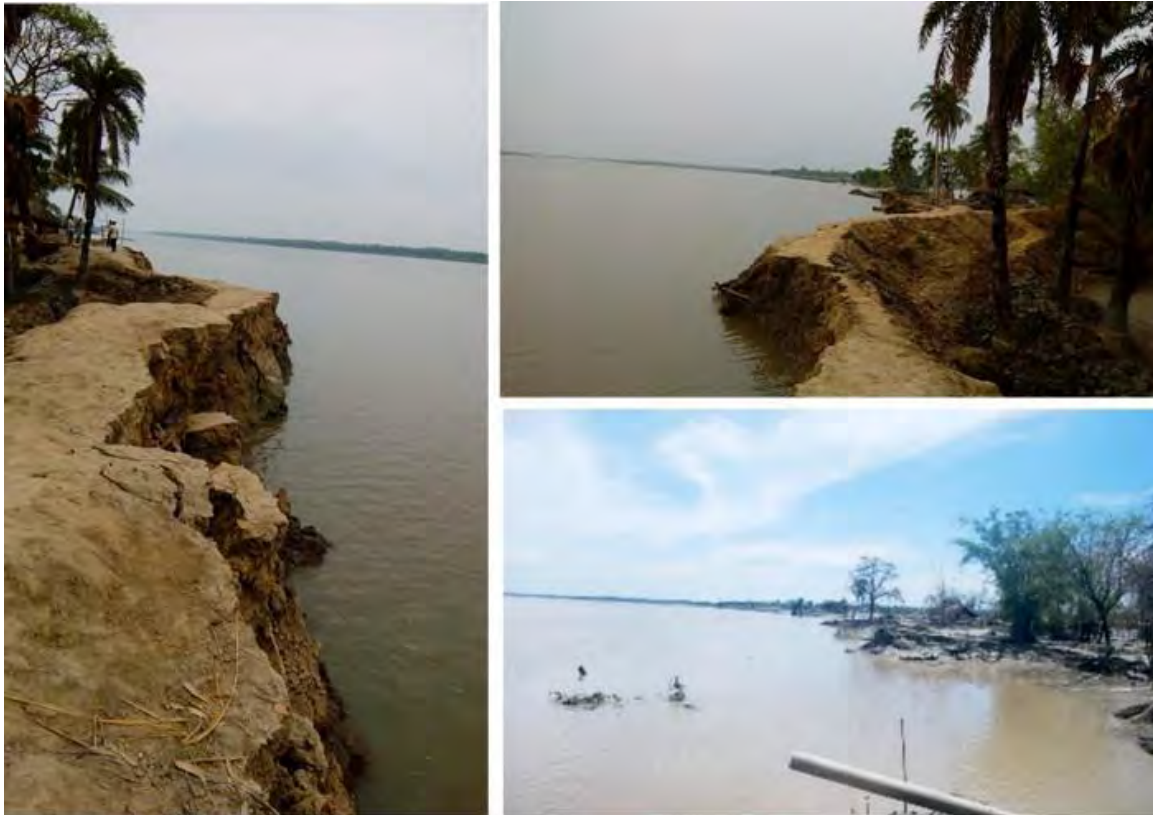
Figure 5.9: Erosion at Polder 29 along Bhadra river
