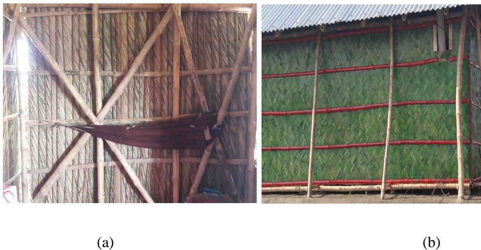
Figure 6.13 Photos of constructed wall structure. (a) Inner portion of the wall consisting bracing against wind force and palm leaves for gathering weight. (b) Outer portion of the wall consisting bamboo matt against surge water and buttress for avoiding lifting.
