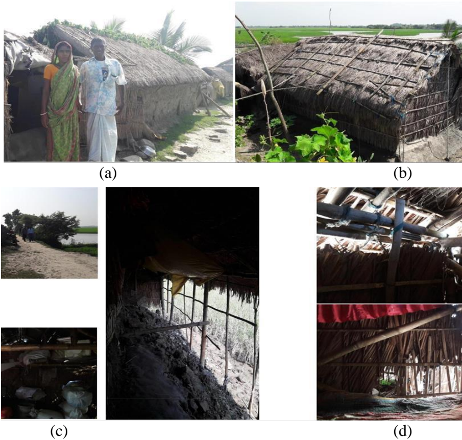
Figure 6.1: Previous housing conditions of beneficiaries. (a) Bikash Roy and Shobita Roy in front of their previous home (b) Bipul Mondol and Lolita Mondol's previous home structure. (c) Bikash Roy and Shobita Roy's home's interior and exterior showing poor physical and spatial conditions. (d) Bipul Mondol's previous home's interior and weak structure.
