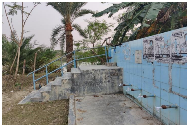
Photo B 4: Non-operational PSF at Sreenagar
