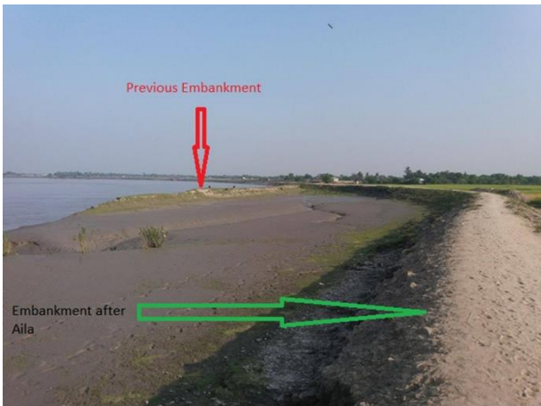
Photo B 1: Breached embankment due to Aila
