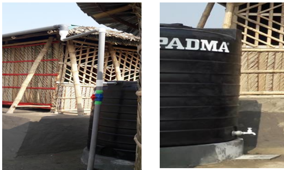
Figure 6.22: Installed water harvesting system in both houses
