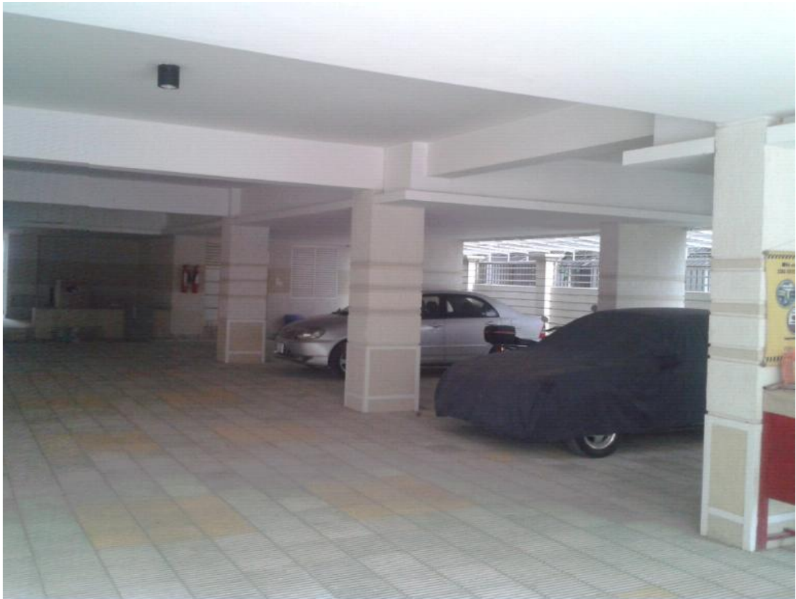
Fig.2.1a A Building with soft ground floor
