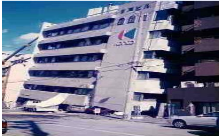
Fig. 2.12 Soft story collapse of the ground floor of a multistoried building; Kobe, 1995
