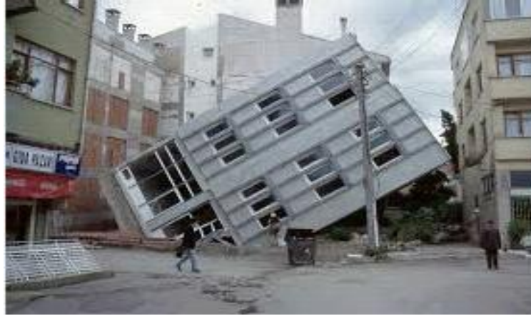
Fig.2.14 Sway mechanisms are often inevitable with soft ground floors; Izmit, Turkey 1999
