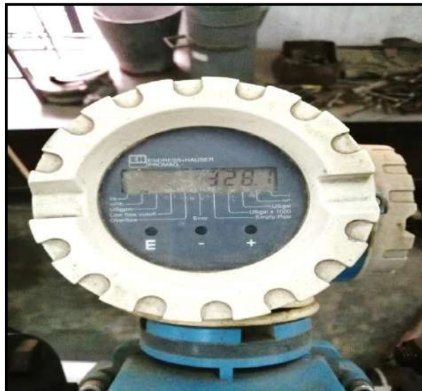
Photograph 3.1: Electromagnetic flow meter.
