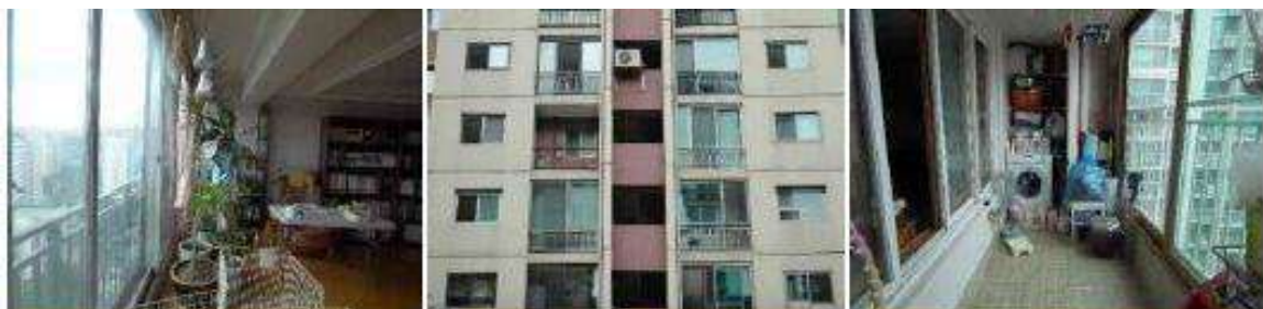
Figure 2. 12: Korean balcony enclosure with sash removal, enclosure with random window frames and enclosure without sash removal (left to right)
