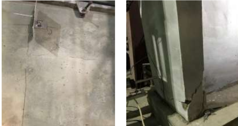
Figure 4.44 Failure modes of wall samples (Hasnat et al., 2022)
