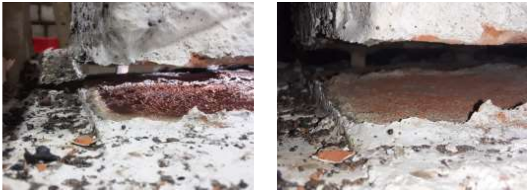
Figure 4.15 Closed view of crack at near end of wall retrofitted directly
