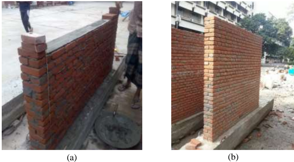
Figure 3.9 Construction of walls, (a) Construction in progress, (b) Fully prepared URM walls
