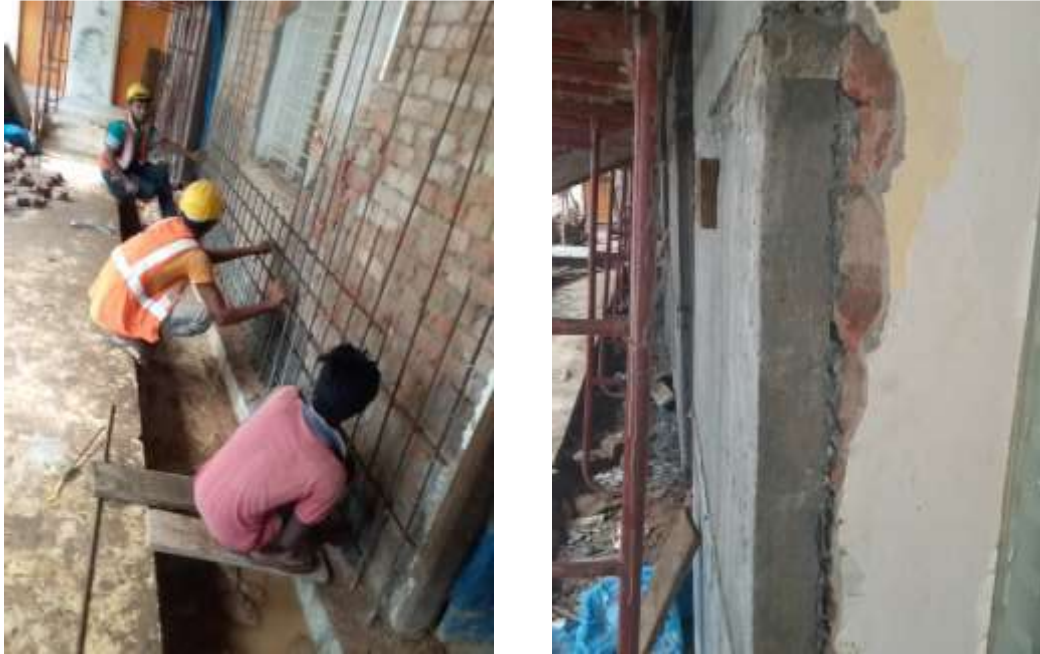
Figure 2.28 Application of RC overlay on the face of URM walls (Retrofitting of DoT building at Tejgaon, Dhaka, 2019)
