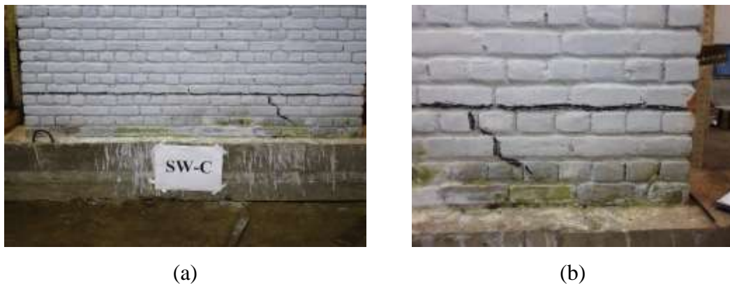
Figure 4.1 Failure patterns in short wall-control specimen (SW-C), (a) Cracks at final stage (4 th cycle), (b) Possibility of toe crushing
