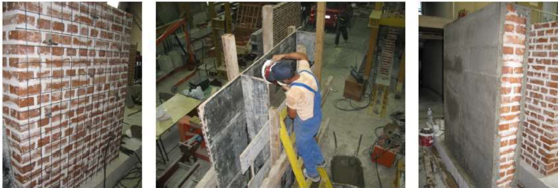
Figure 2.37 Application of RC jacket on both sides of the wall (Sergey and Elena, 2011)
