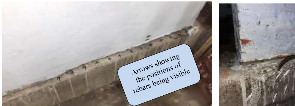
Figure 4.11 Near end of LW-CR wall lifted up from base
