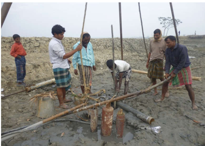
Figure 3.4: First borehole, BH-1 (21.5 m deep), near old embankment at Patakhali closure, Koyra, Khulna.
