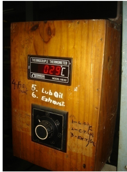
Fig 3.38 : Temperature measuring unit.
