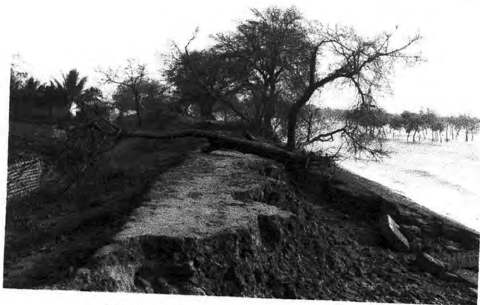
Photo of Damage Road Casualty
