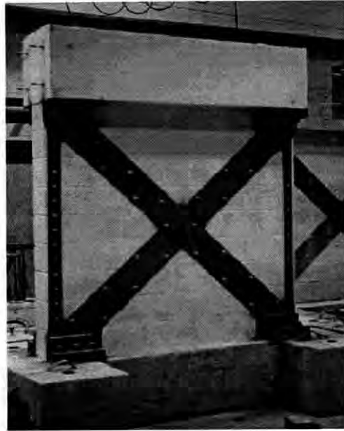
Fig. 2.1. The steel strip retrofitting techniques suggested by Taghdi et al. (2000) for unreinforced masonry walls
