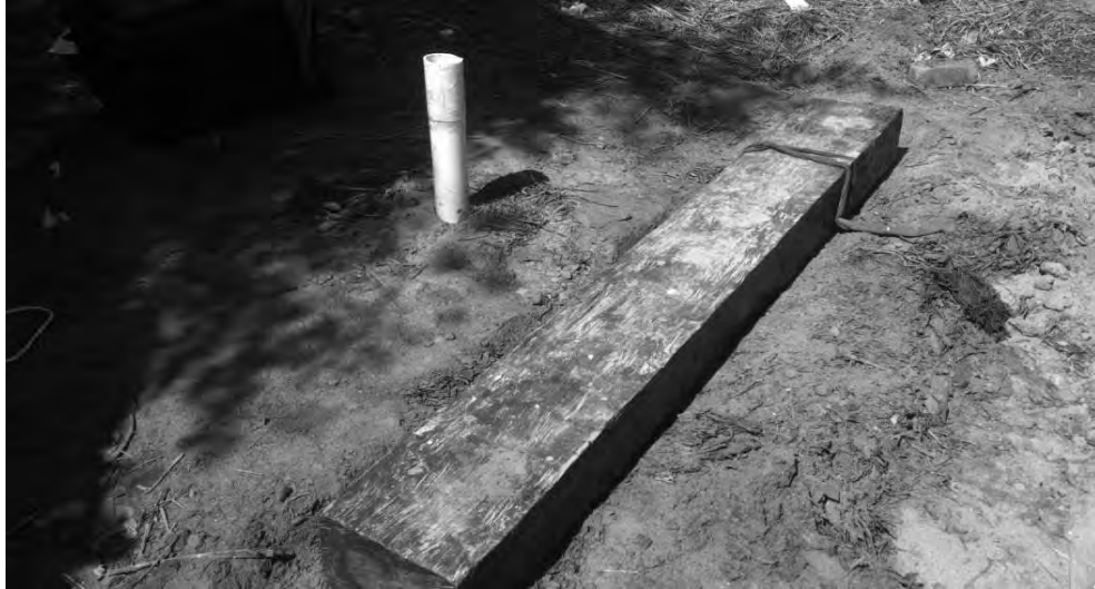
Figure 3.6 A heavy wooden plank used for PS Logging Test at Kamrangichor, Dhaka
