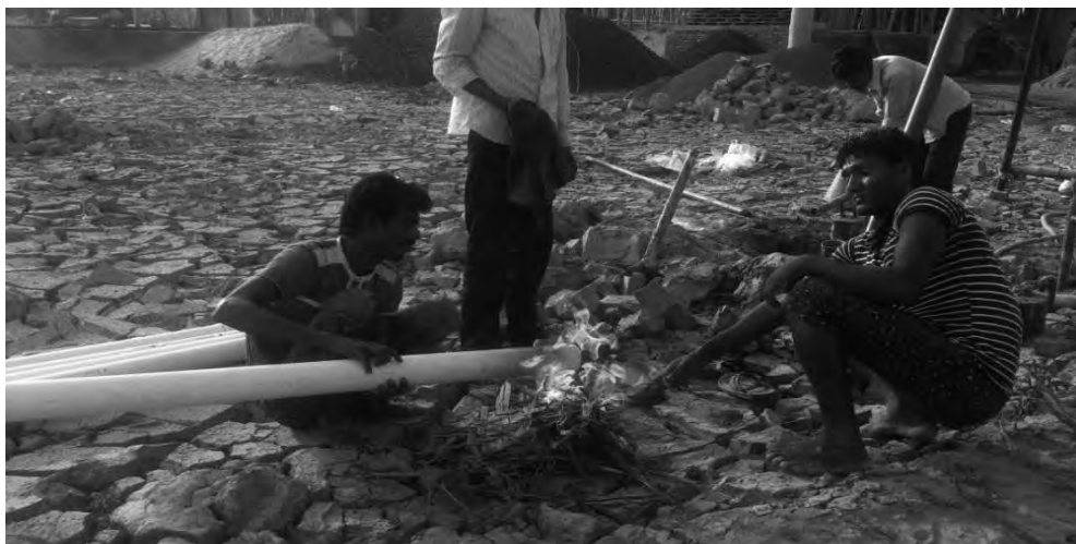
Figure 3.4 Burning of PVC pipe at bottom, before installation
